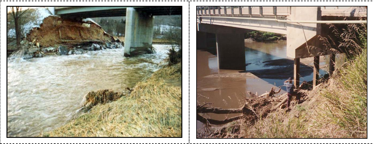
Figure 1. Abutment failure due to scour typically is attributable to the geotechnical failure of the abutments spill-slope, as illustrated by these two examples.
